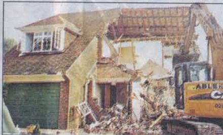
RELIC: The Hayeses knocked down this Sixties house to make way for The Grange
